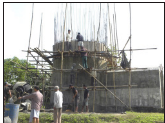
Construction of base for ‘Shanti Doot’ under progress at the SACH cultural complex.
